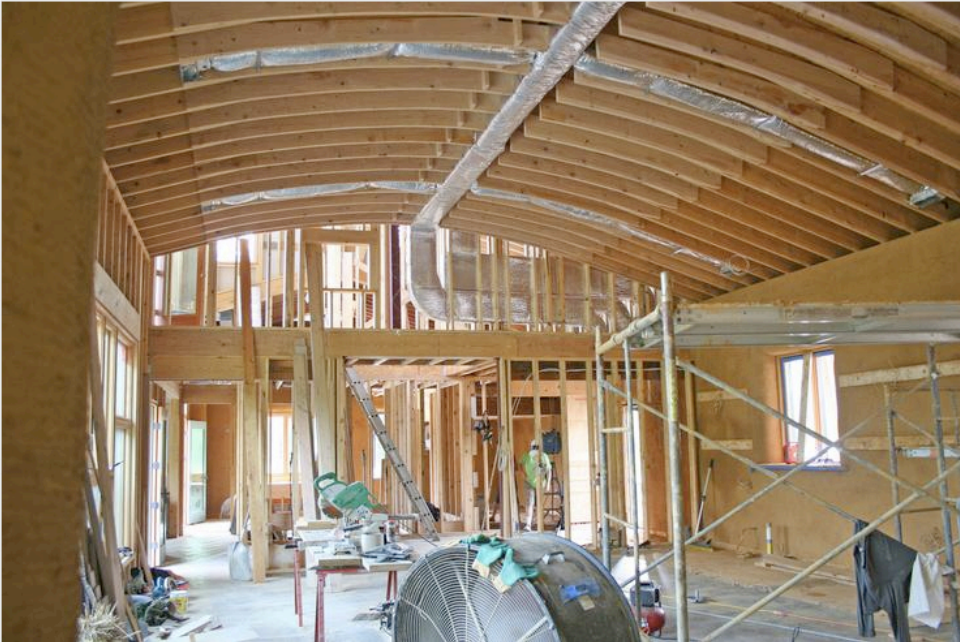
The interior of the house consists mostly of a two-story great room with a barrel-vaulted ceiling. The space will be heated and cooled by geothermal wells and passive solar design.
