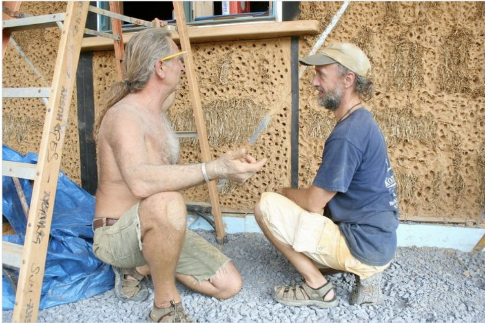
General contractor Gary Stiewing, left, examines a section of straw-bale wall laid by Steve Kemble of MudStrawLove. Kemble's firm built the super insulated walls with help from 12 volunteers.
